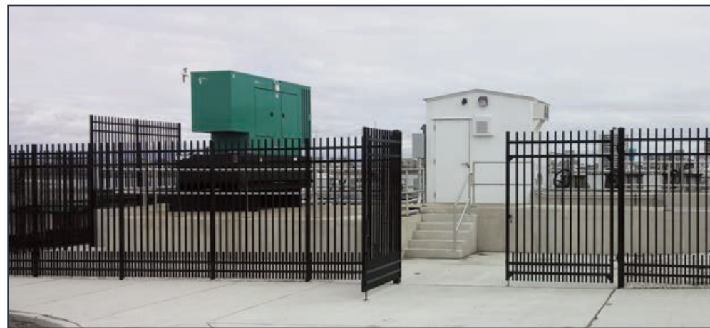
Ventnor Gardens Pump Station, Ventnor City (Source: ACUA - Ventnor Gardens Plaza Stormwater Pump Station Fact Sheet)
