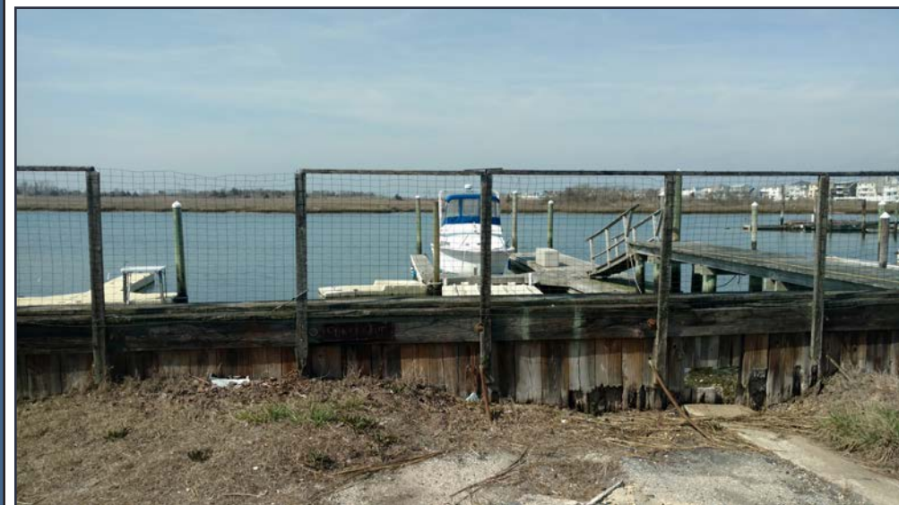
Damaged Back Bay Bulkhead
